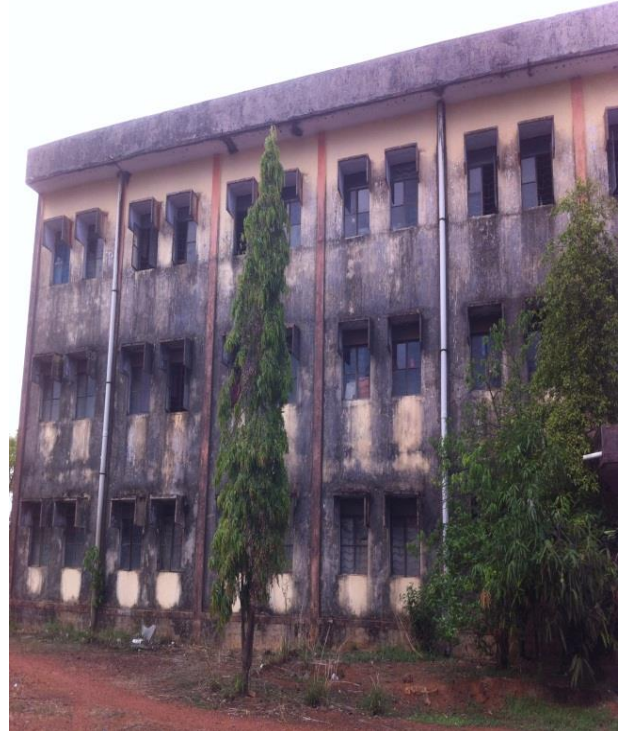
Painting and maintenance required in WWH, Academy of General Education, Udupi
