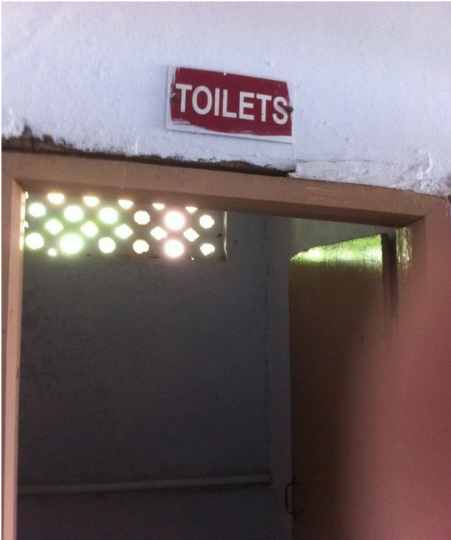
Door frame separated from the wall in JSS Vidyagiri, Dharwad
