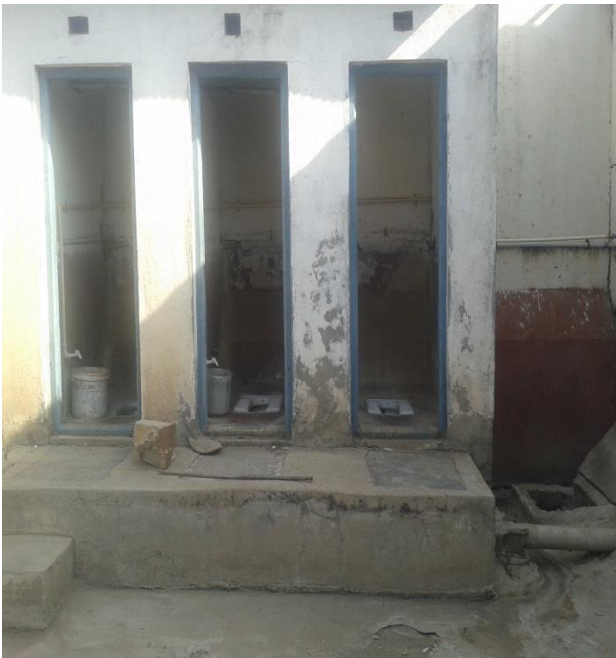
Maintenance required in toilets at Sri Basaveshwara Vidya Vardhaka Sangha WWH, Bagalkote
