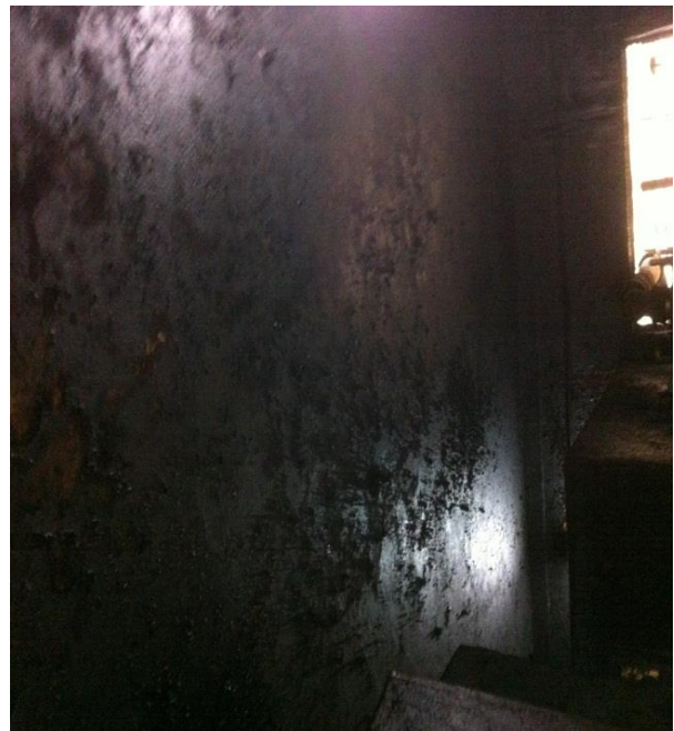
White washing of walls required in Kasturba Sadanand WWH, Chikmagalur
